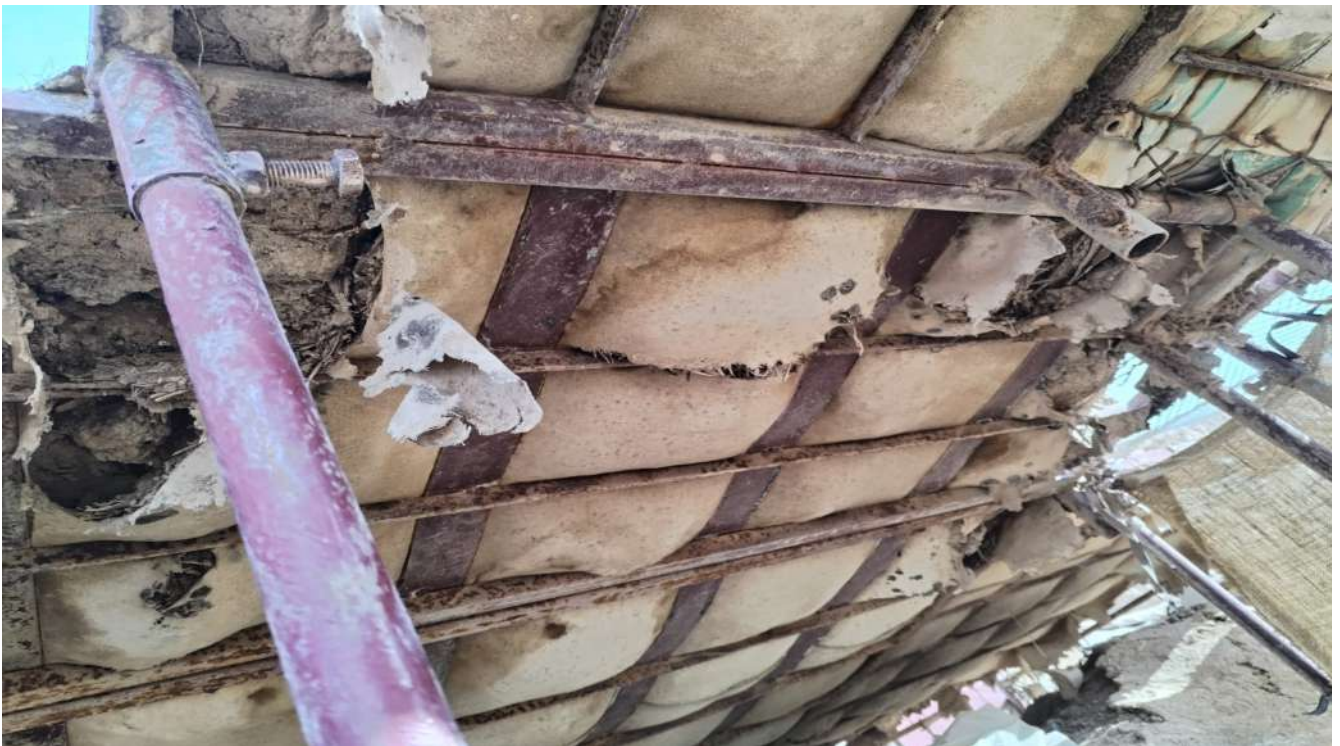
Figure 8: An image illustrating signs of deterioration in the burlap
