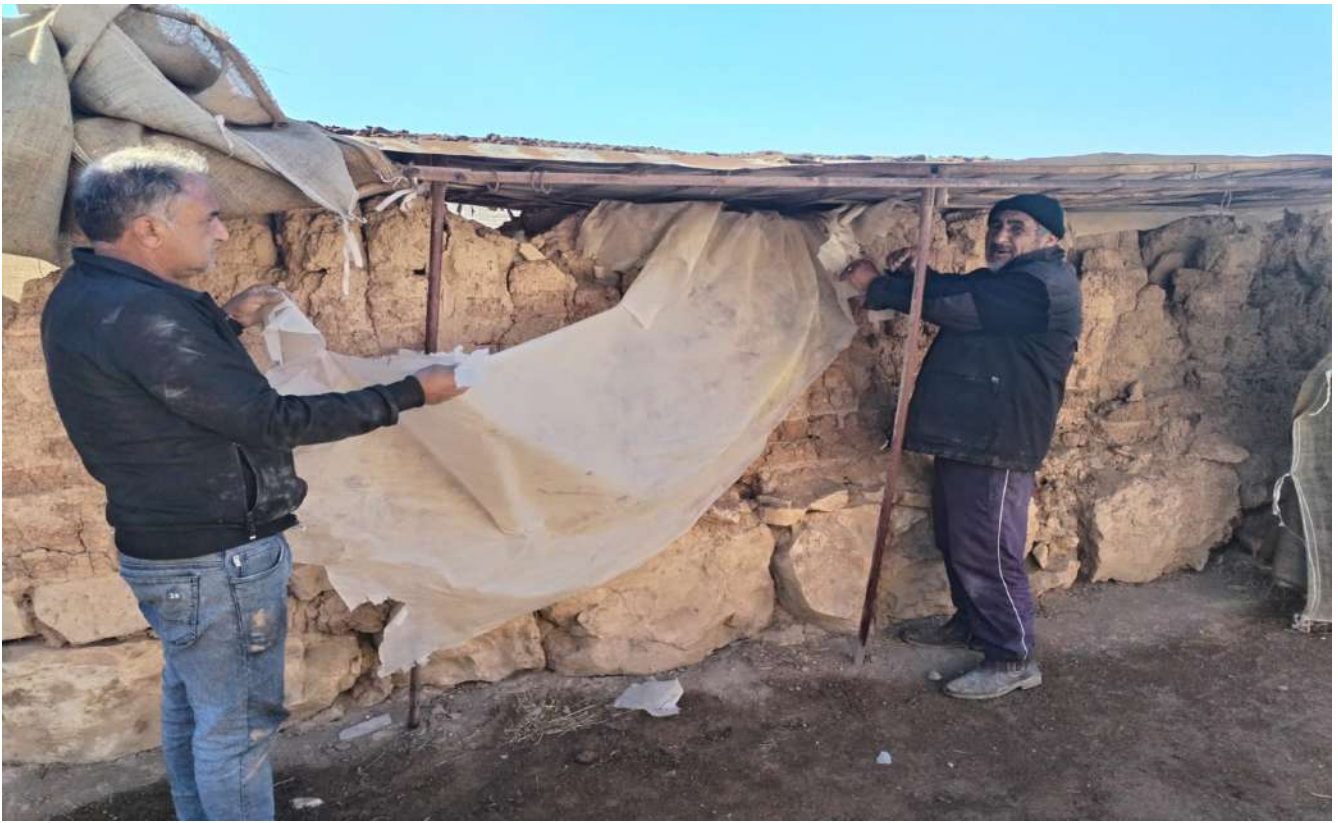
Figure 31: Torn and worn nylon over the walls
