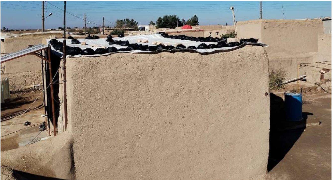
Figure 17: Type of plastic sheet used to cover local mud-brick houses in Mozan village
