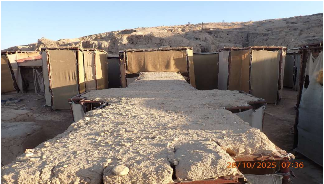
Figure 27: Mud plaster condition in service wing
