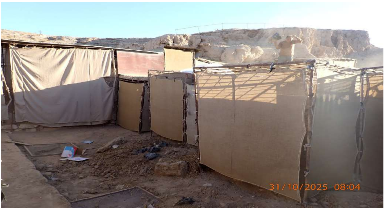
Figure 12: Debris accumulated at the base of the walls and on the room floors
