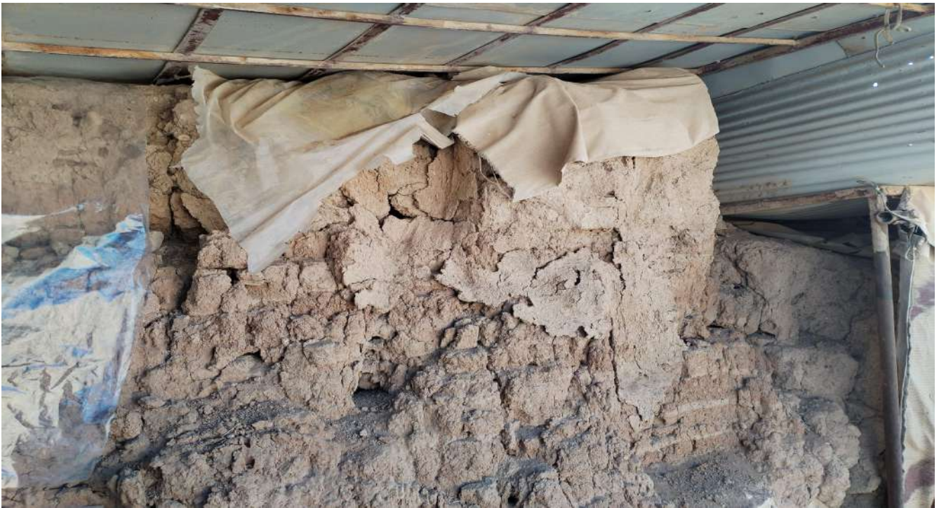
Figure 21: Contact of the sheet metal (tutiya) surface with the top of Wall F1-4 (center)
